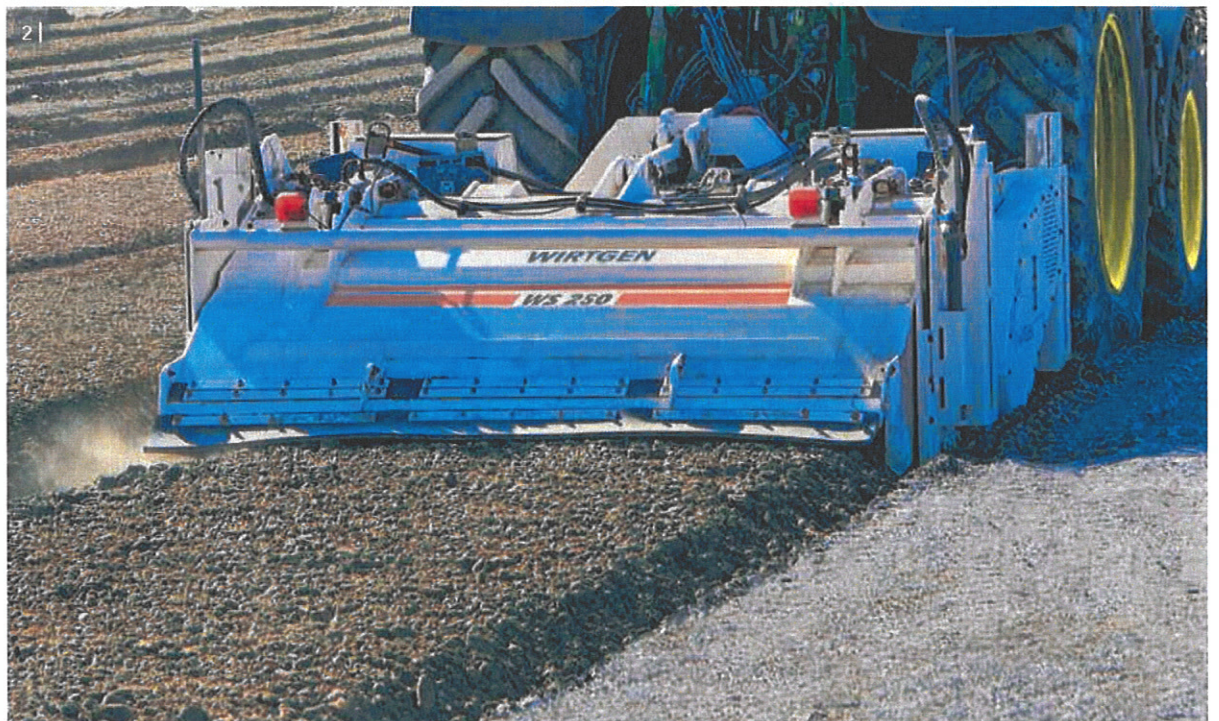
2 | Flawless mixing results and perfect leveling are the hallmarks of the tractor-towed stabilizer.
